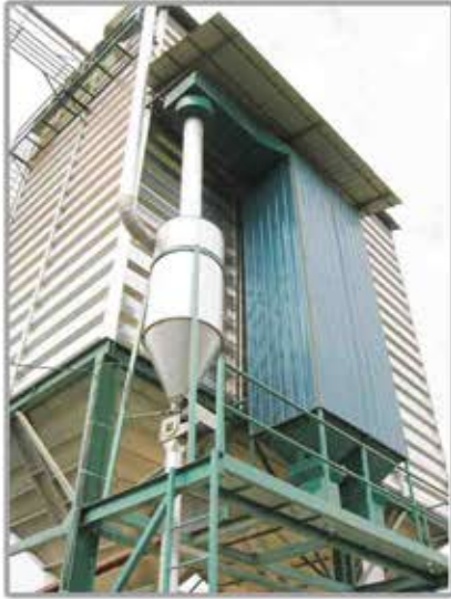
Air exhaust through cyclone and filter bag.
