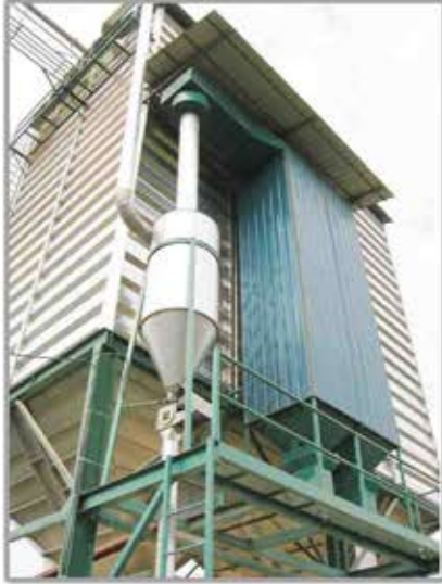
Air exhaust through cyclone and filter bag.
